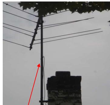
Unused antenna should be removed, to decrease resistance on chimney.
