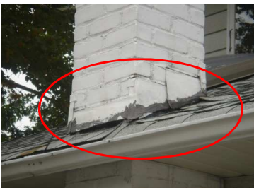
Flashing around chimney needs immediate attention.
